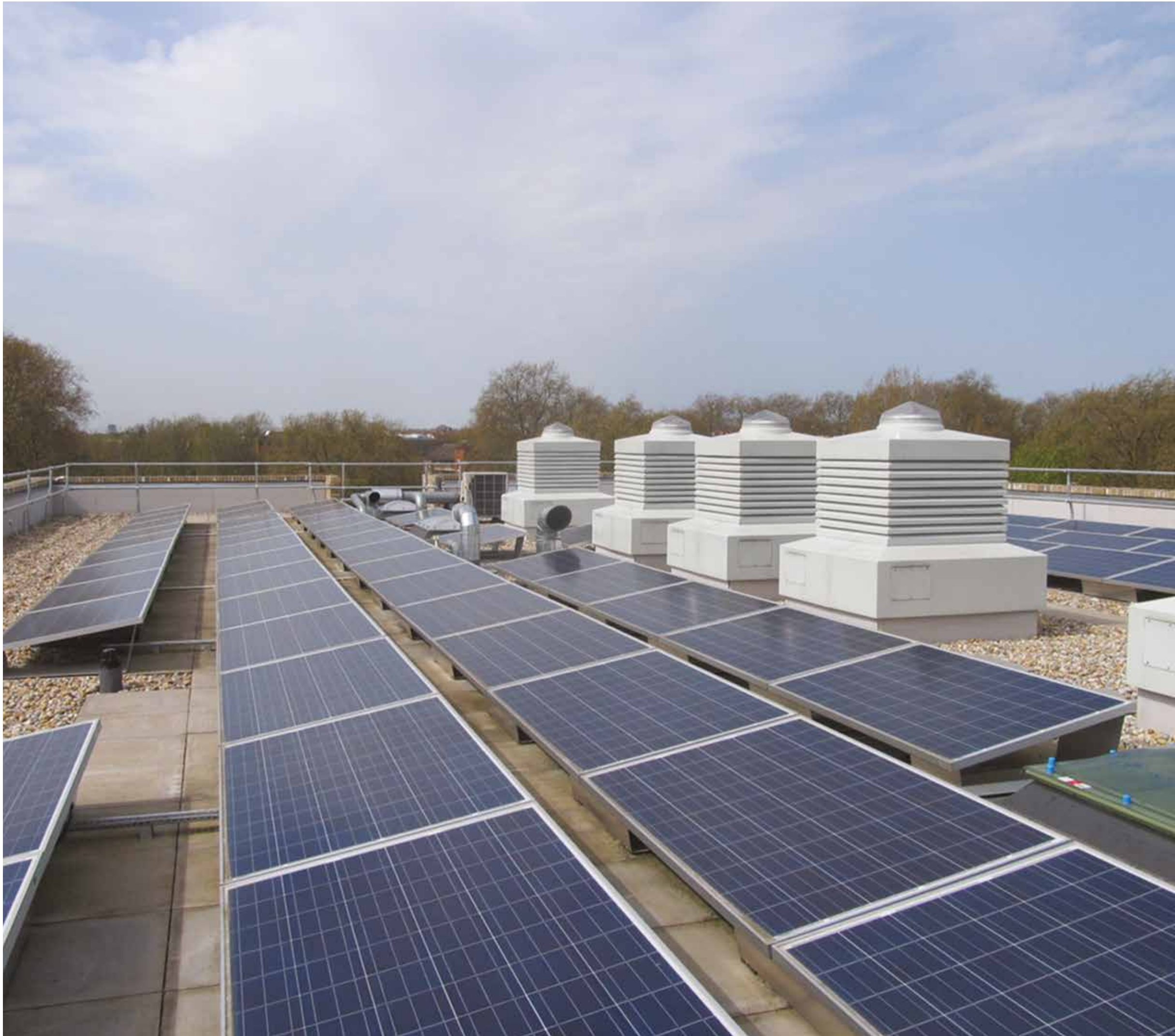
Example image of solar panels
