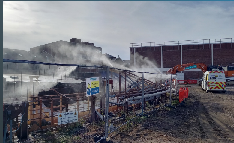
Odour suppression on venting gas holder.
